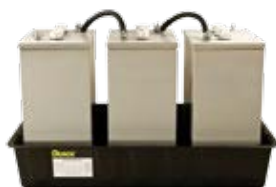
Battery tray with three L16/GC2 batteries 120221
